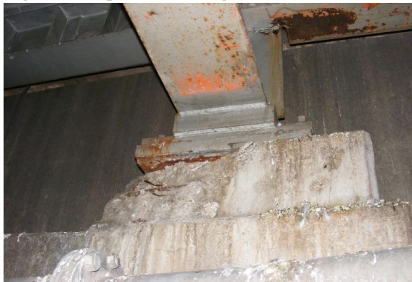
Figure 11 [Spalled Bearing Pad]
